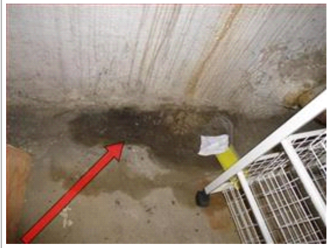
Active water leak noted at water meter fitting. Recommend: Qualified Plumbing Contractor Repair/Correct.
