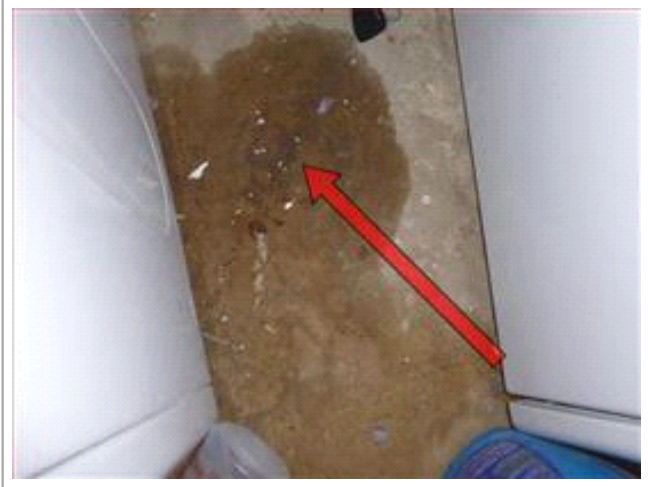
Water leak evidence noted in basement from bathroom piping above. Recommend: Qualified Plumbing Contractor Evaluate/Repair/Correct.
