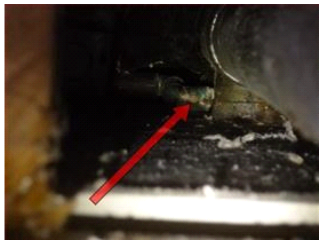
Water leak evidence noted in basement from bathroom piping above. Recommend: Qualified Plumbing Contractor Evaluate/Repair/Correct.
