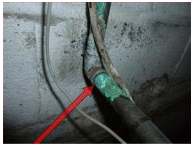
Active water leak noted at water meter fitting. Recommend: Qualified Plumbing Contractor Repair/Correct.
